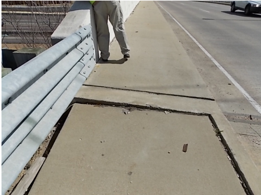
APPROACH 1 LEFT SIDEWALK SETTLED
