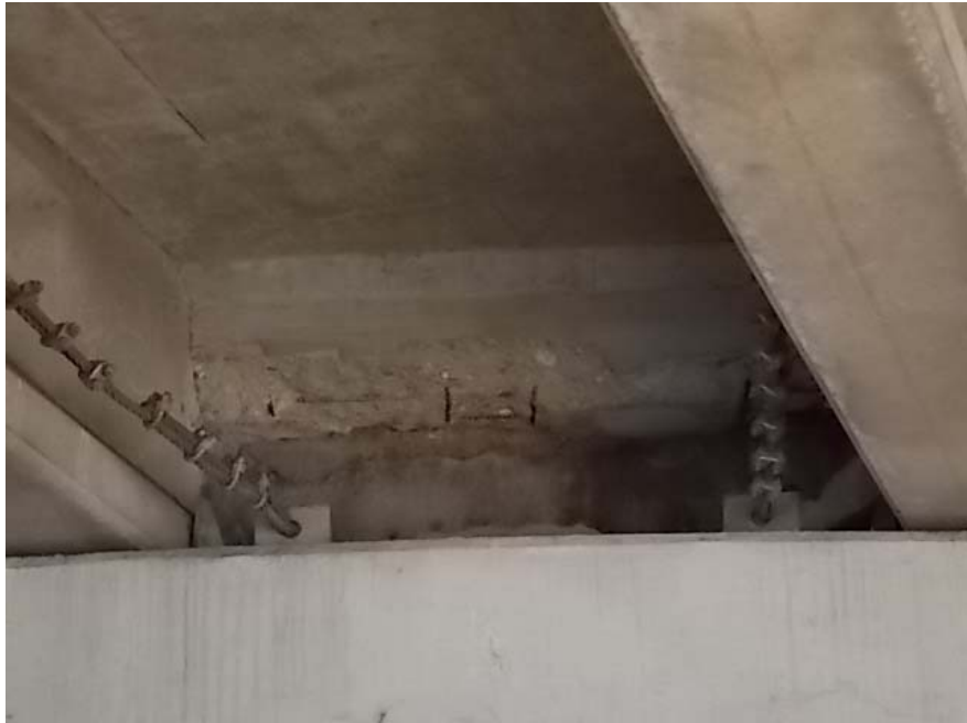
SPAN 5 DIAPHRAGM SPALLING
