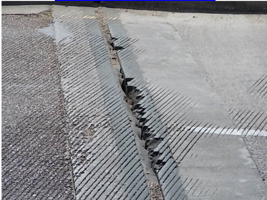
SPAN 5 JOINT SPALLING
