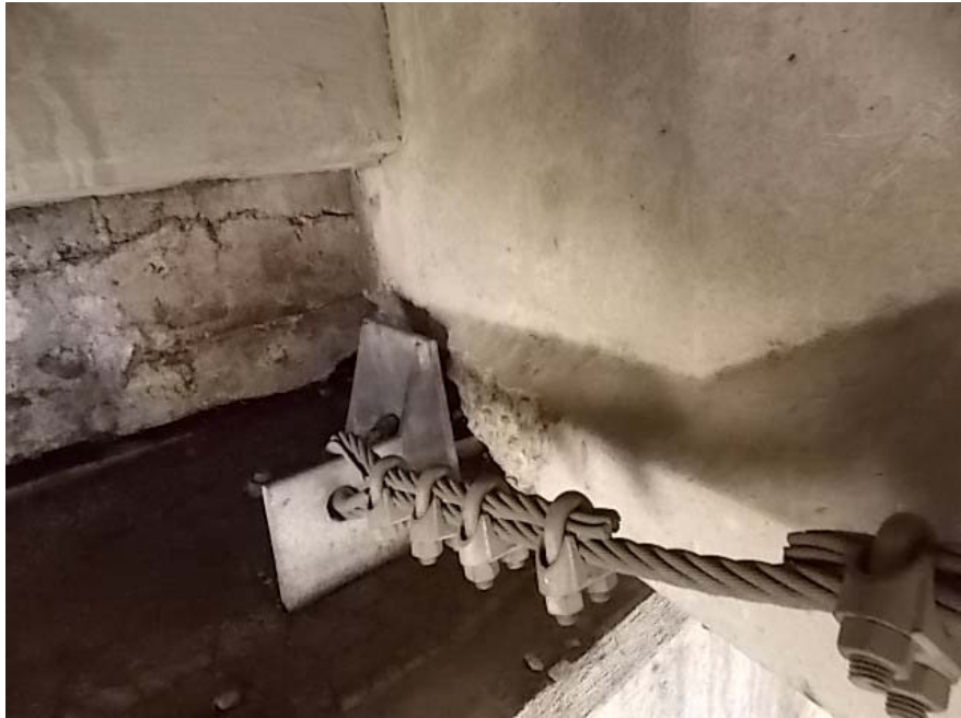
SPAN 5 BEAM C SPALLING
