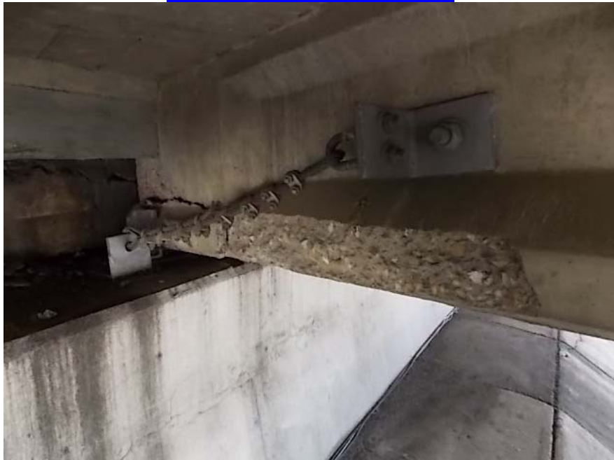
SPAN 5 BEAM D SPALLING
