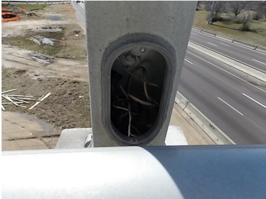
SPAN 5 COVER PLATE MISSING ON LIGHT
