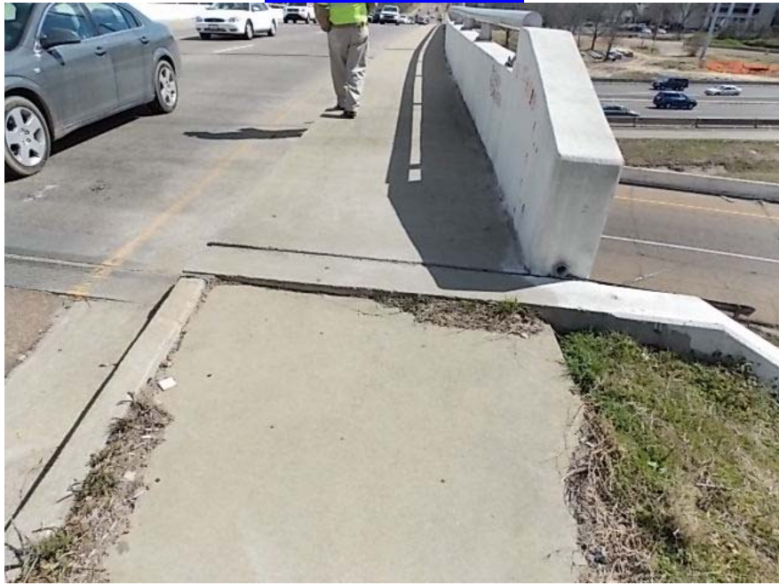
APPROACH 1 RIGHT SIDEWALK SETTLED
