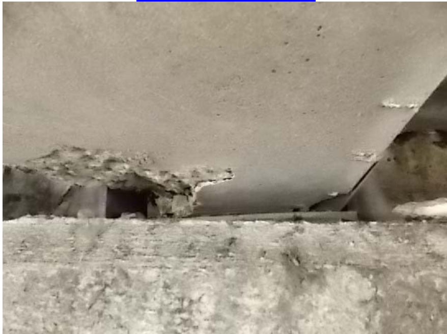
SPAN 5 BEAM C SPALLING
