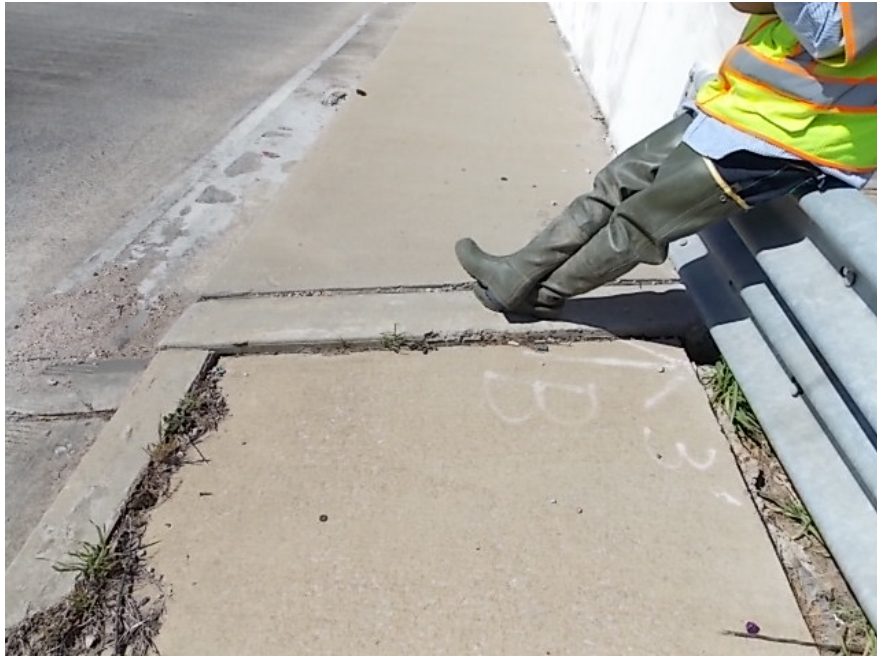
APPROACH 2 LEFT SIDEWALK SETTLED
